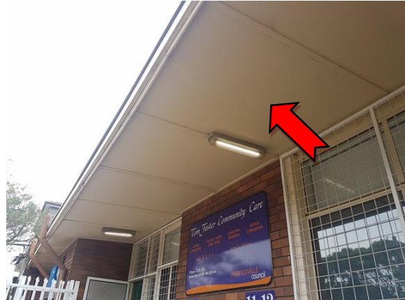
Photo 2. Exterior, south-west elevation, awning – suspected asbestos-containing fibre cement sheeting.
