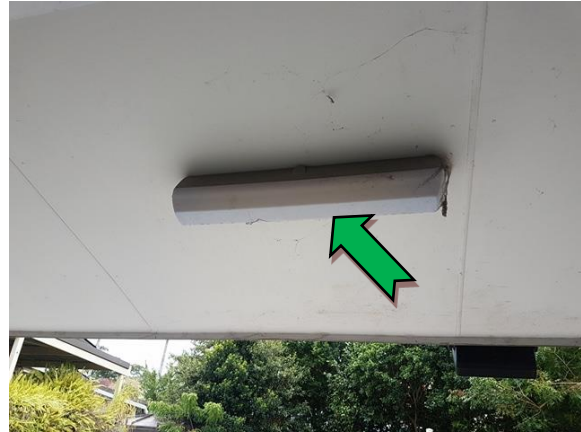
Photo 14. Exterior, throughout, single tube fluorescent light fittings – suspected non PCB-containing capacitors.
