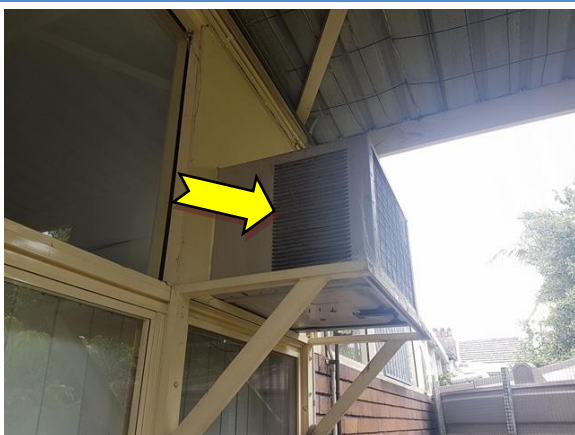
Photo 17. Exterior, north-east elevation, air conditioning unit, unknown refrigerant – suspected ozone depleting substance.
