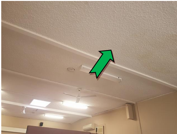
Photo 9. Interior, north-west elevation, dining hall, ceiling – non asbestos-containing sprayed vermiculite.
