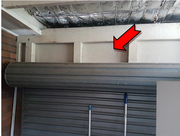
Photo 7. Interior, store room/garage, infill panels – suspected asbestos containing fibre cement sheeting.
