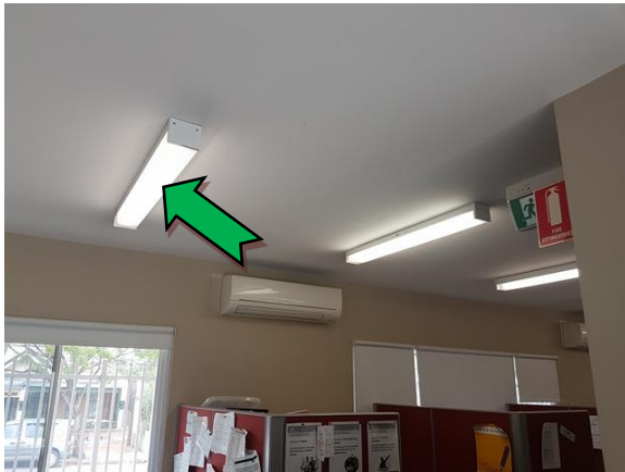
Photo 15. Interior, throughout, double tube fluorescent light fittings – suspected non PCB-containing capacitors.
