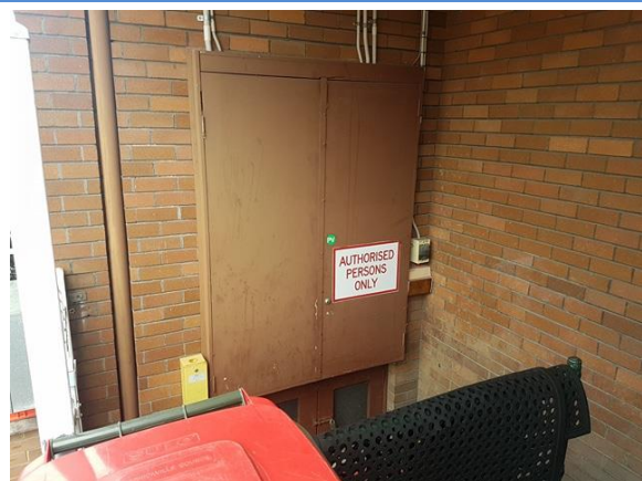
Photo 18. Exterior south-west elevation, electrical distribution board – no access at the time of assessment.
