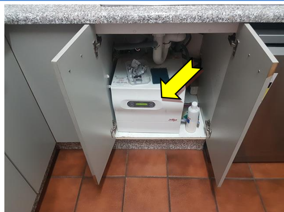
Photo 12. Interior, kitchen, under sink, hot water heater – suspected SMF internal insulation.
