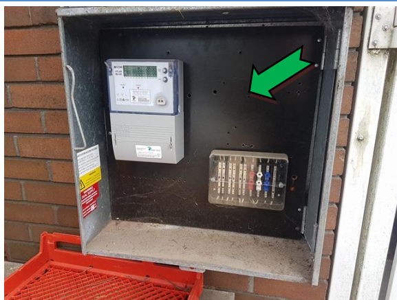
Photo 5. Exterior, south-west elevation, electrical backing board – suspected non asbestos-containing bituminous backing board.
